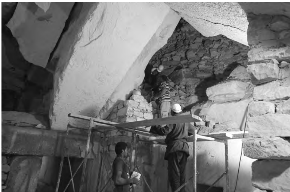
Fig. 17 The consolidation works of the eastern wall of the antechamber (photo M. Megahed)
